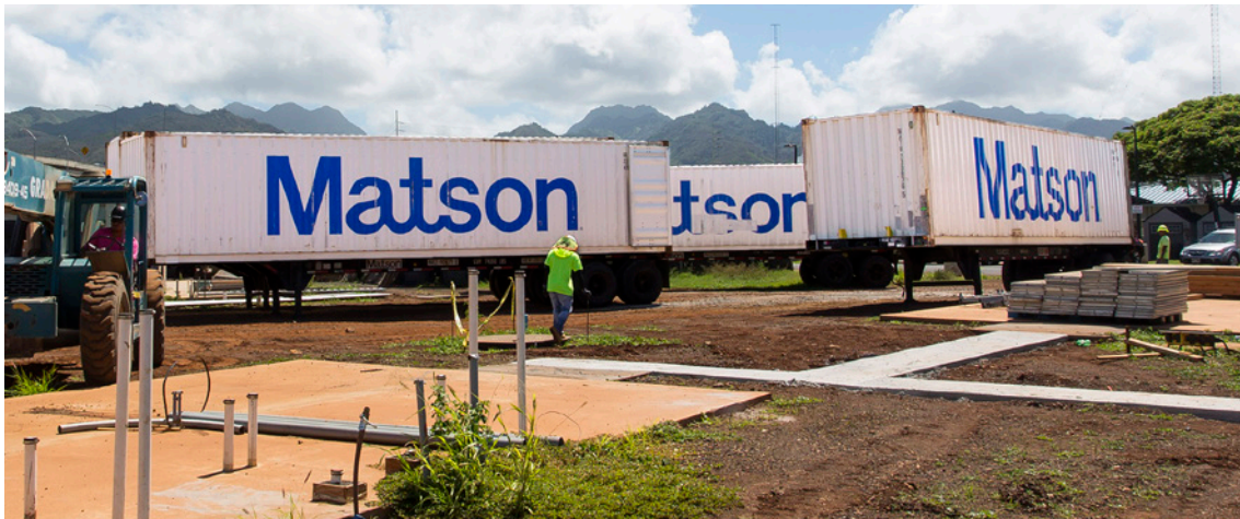
At the Kahauiki Village site, these Matson containers are filled with prefabricated homes, sourced from Japan by aio Foundation and shipped to Oahu at no charge. The homes will be assembled on the concrete foundations which are prepared with electrical and plumbing rough-ins. Long-term affordable housing will help break the cycle of homelessness.
